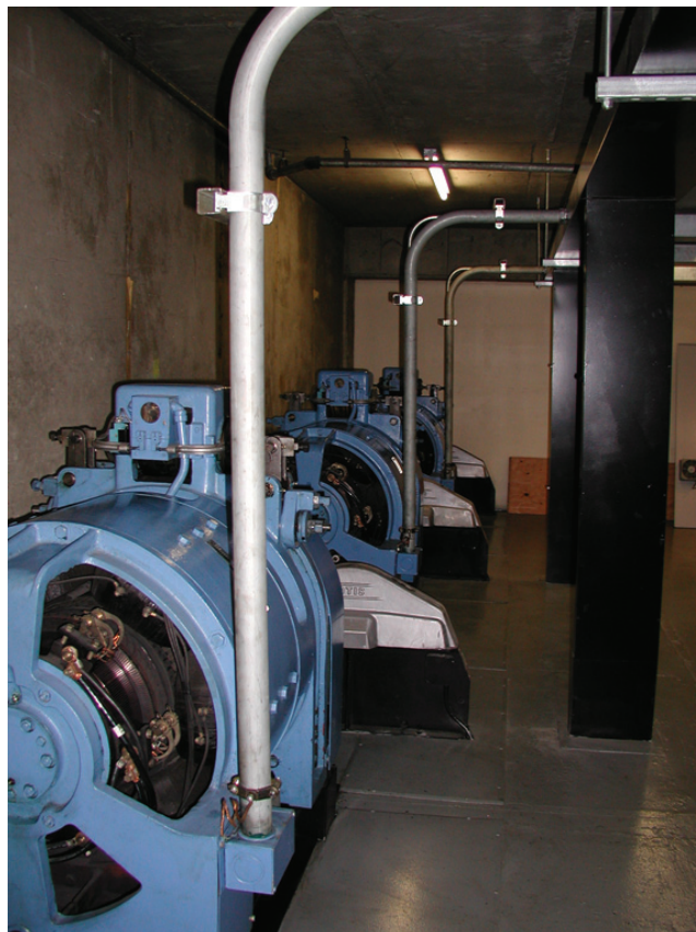
Otis DC elevator motors
