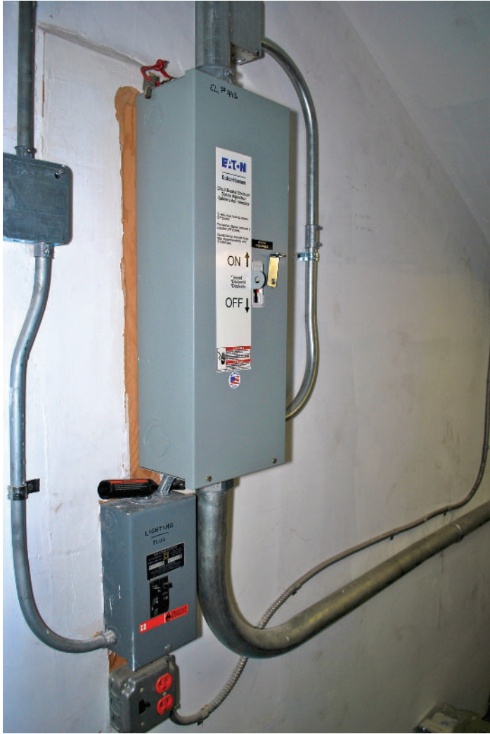
Power coming into the machine room with a ground-fault circuit interrupter-protected receptacle on a dedicated circuit as required.
