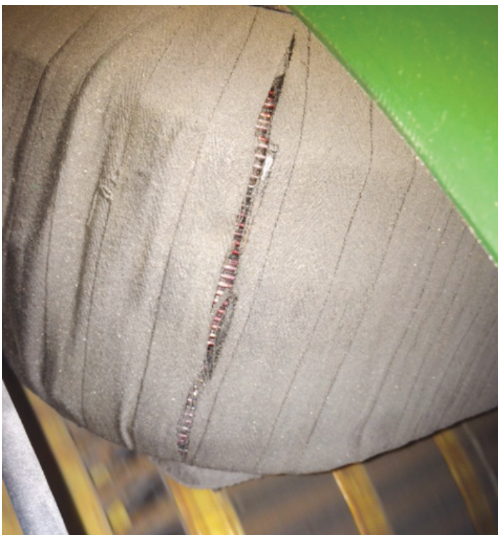
The cracks in this machine's coil insulation can easily be overlooked, as replacement costs thousands of U.S. dollars.
